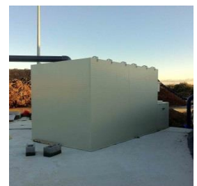
Filter of exhaust air: Bio filter + active coil filter
