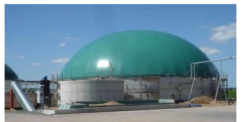
In the foreground : solids dispenser In the middle: cesspit In the background : digestate storage
