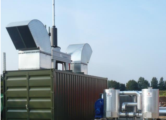
CHP-Unit in Container
