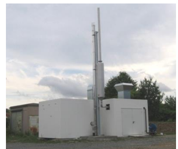
CHP-Unit in garage
