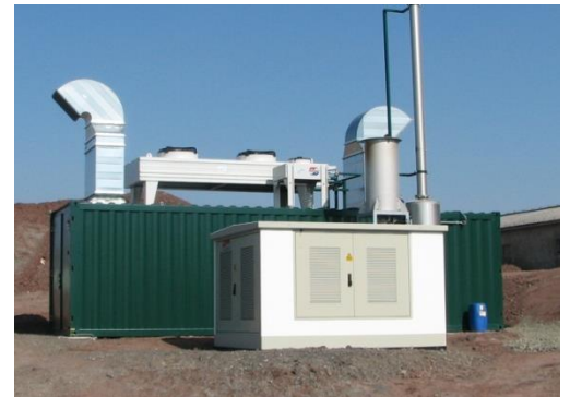
CHP-Unit in Container In the foreground: transformer station
