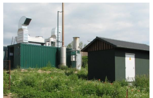
CHP-Unit in container and transformer station
