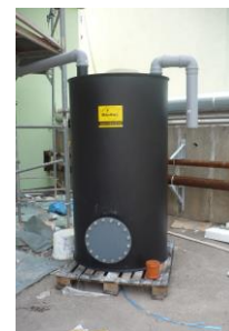
Desulphurisation of the gas
